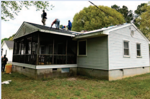
The roof on this home in Melfa was replaced through qualified USDA funding.
